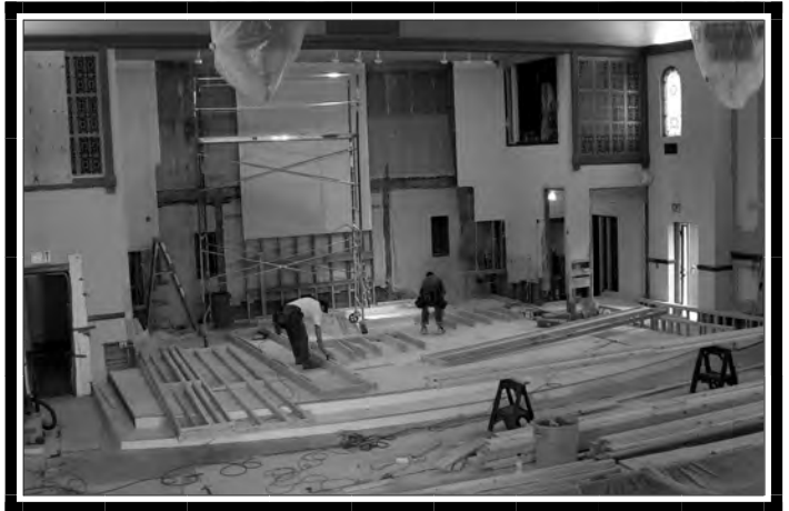
View from the balcony as the workers are building the sliding doors of the dossal
